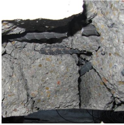
a) photo of failed rebar in PGEDB2
